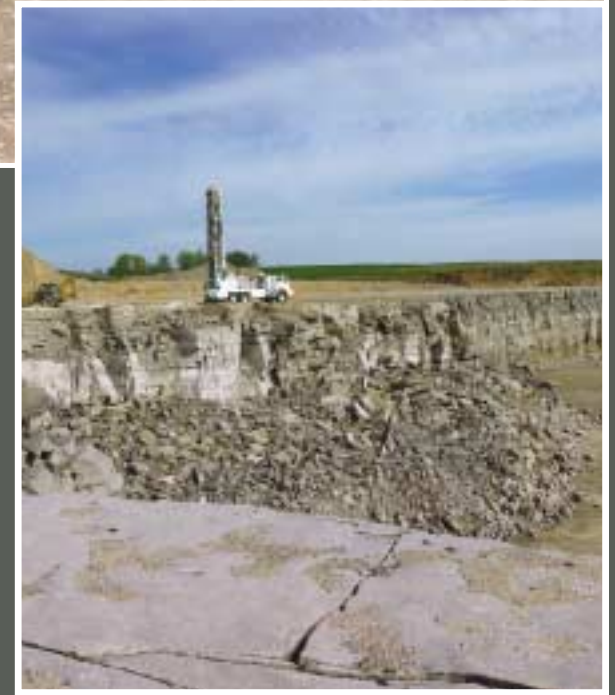
A drilling rig is used to bore holes into the limestone. Explosives are then placed and the blast detonated from the other side of the quarry.
