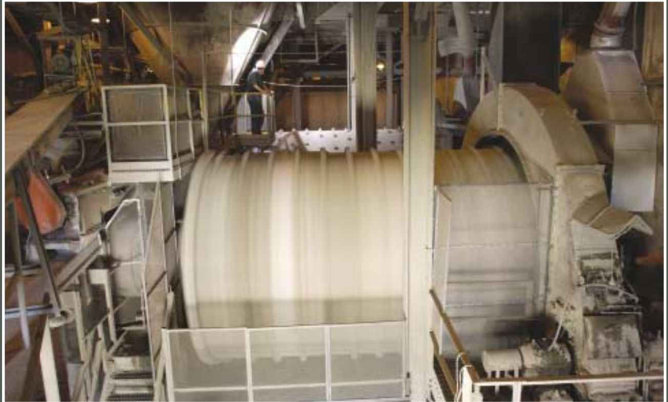
Ball mills (five all together) are essentially steel tubes which contain various sized steel balls. As the mills rotate, the clinker is crushed into a fine powder.
