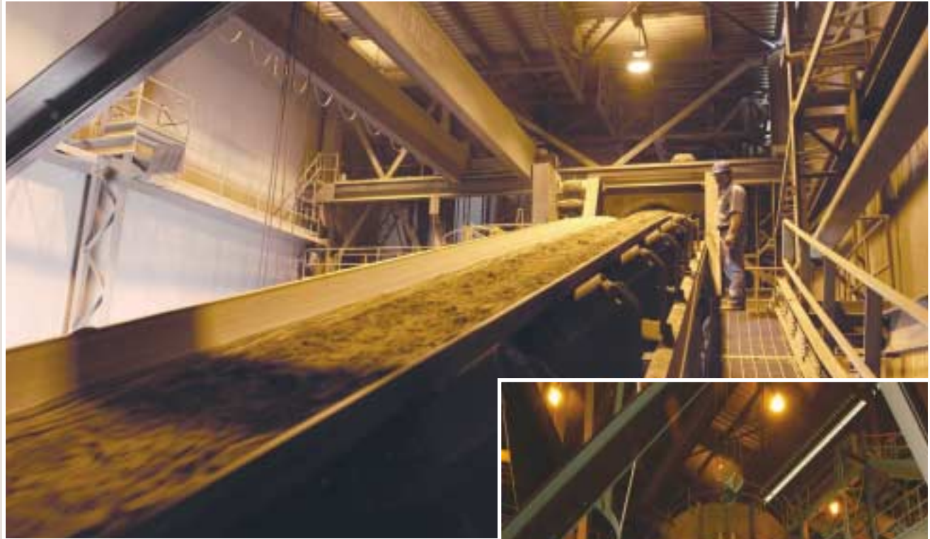
Gary Smale watches the roughly two-to-one mixture of limestone and clay on its way from the raw mill.
