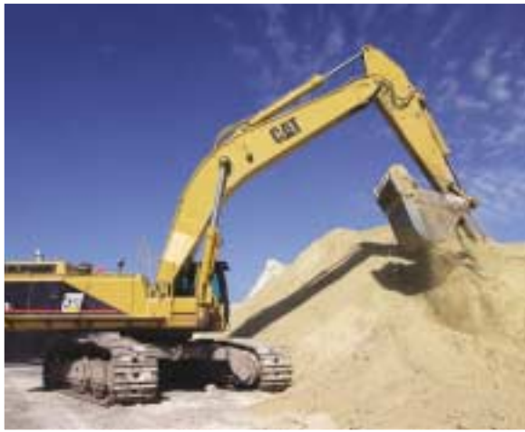
A Cat 375 backhoe digs deep into a pile of silica, one of the raw materials required to chemically balance the manufacture of Portland cement.
