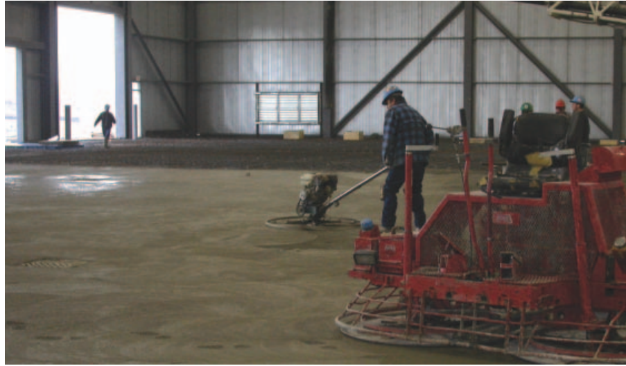
Even in freezing temperatures the finishers were able to get off the floor the same night.
